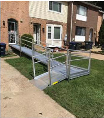
This ramp was for three stairs, approximately 21" in rise.
